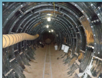
Tunneling operation to install a new 72-inch RCP under the CapMetro Redline
