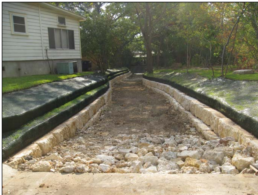
North Fork Tributary of West Bouldin Creek at Manchaca Road Channel Rehabilitation
