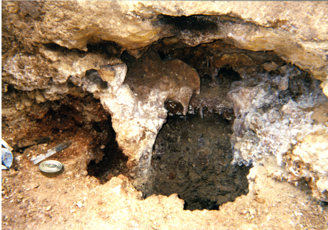
Four Points EMS/ Fire Station, void C
