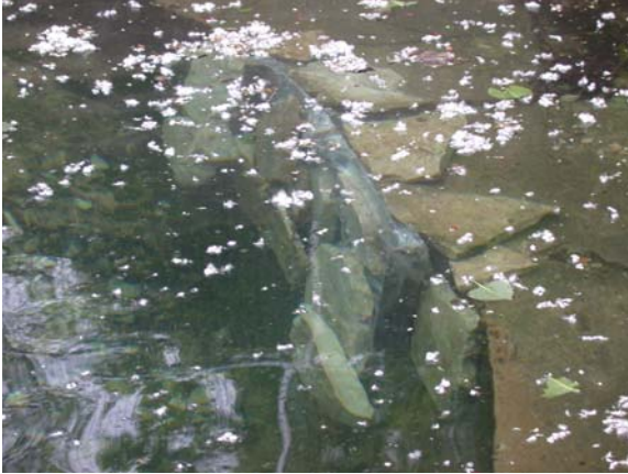
A) Blocked Grate
