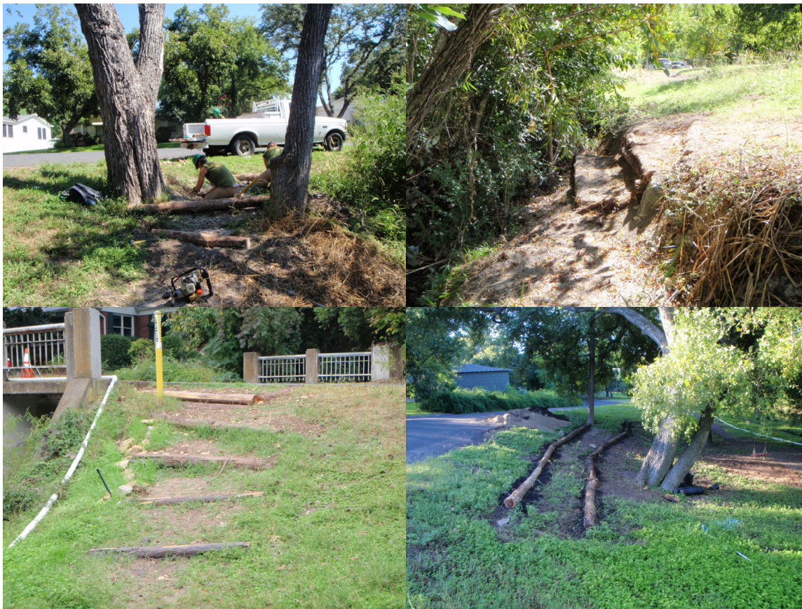
Figure 3. Examples of hardscaping installed by AYW include juniper log access steps and terraces to prevent street from street runoff.
