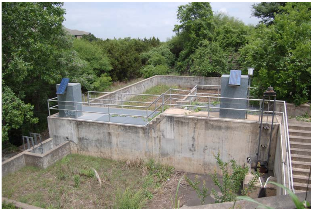
Figure 93 Photograph of the Barton Ridge Sand Filter
