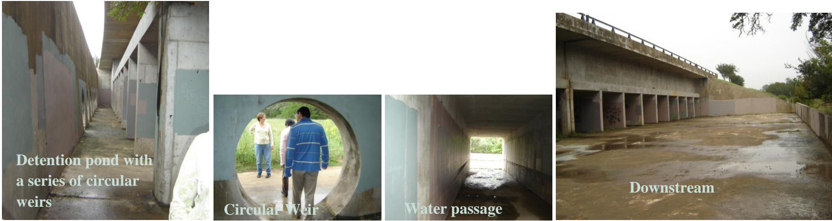
(b) Detention Pond-Type 2 with multi-stage circular weir for flow control
