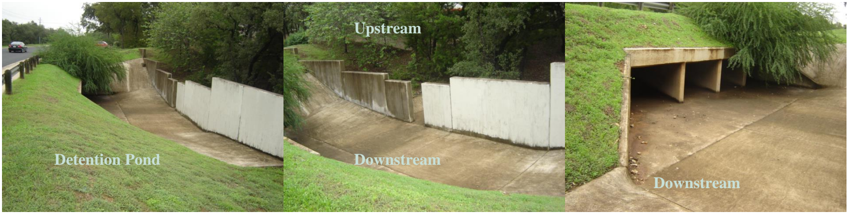
(a) Detention Pond-Type 1 with stepped rectangular weir for flow control
