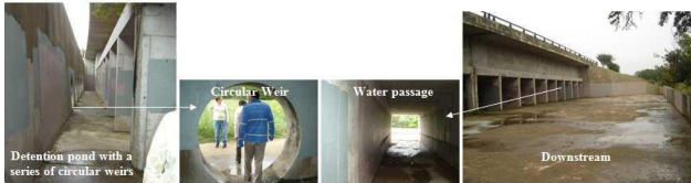
Figure 1b Detention Pond-Type 2 with multi-stage circular weir for flow control (Courtesy: City of Austin, TX)
