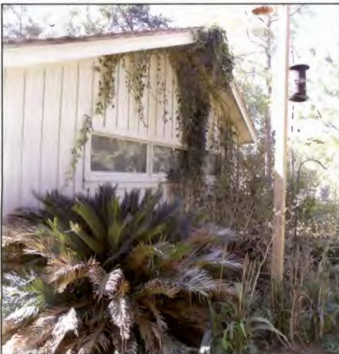
Overgrown vegetation that is within the 30 feet of defensible space can produce significant heat, potentially igniting the home.
