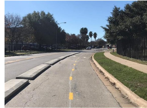
Elmont Dr to Riverside Dr Two-way protected bikeway with barrier curb + sidewalk
