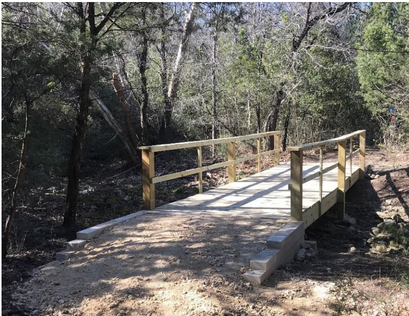
The Texas Conservation Corps built this pedestrian bridge on the Snowden tract along a trail that is used for guided hikes. This bridge also provides utility vehicle access between the Natural Resources Field Office and the Snowden House.
