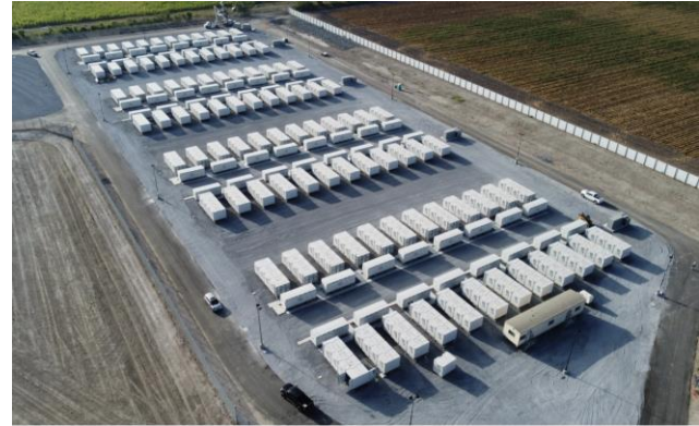
Eolian LP's Madero & Ignacio 200 MW energy storage project
