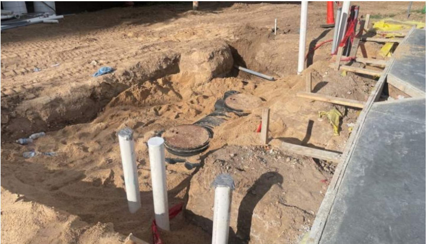
South Building Addition: Grease trap.
