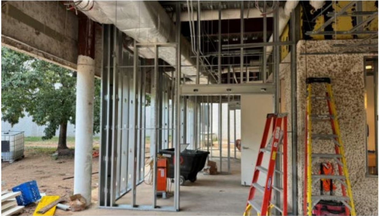
Building: Metal stud framing of new partitions or walls for new Youth Offices.
