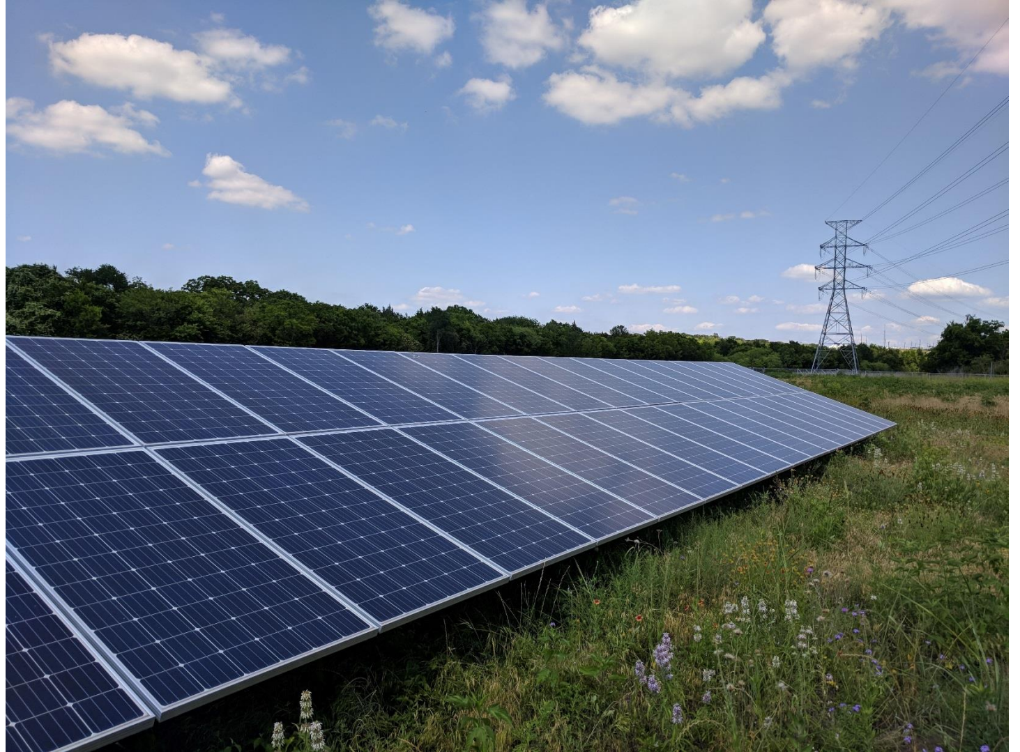
La Loma Community Solar Farm
