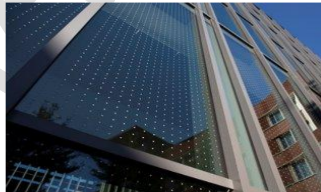
Figure 3. Example of glass frit, from Google building in downtown Austin. Photo by WPD staff.
