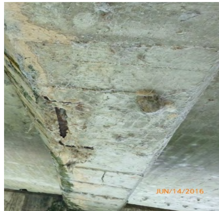
Longitudinal Beam - Exposed Rebar
