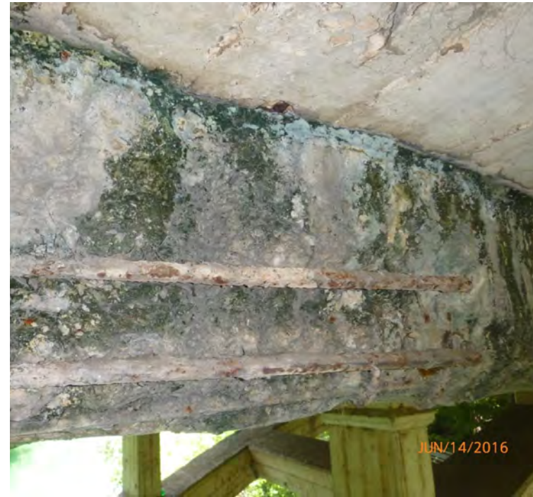
Longitudinal Beam - Exposed Rebar
