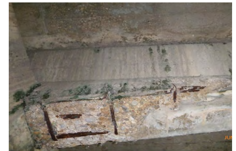
Exposed Rebar, Degraded Con
