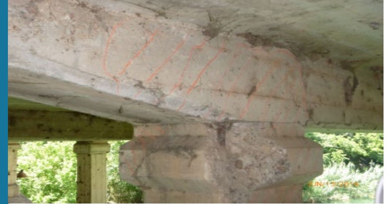
Delamination of Beams
