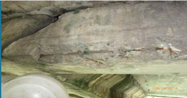
Spalling Concrete in Bridge Structure
