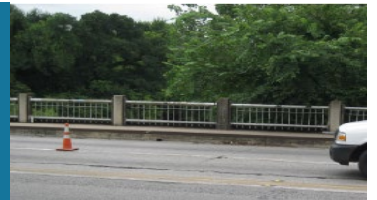
Curb And Railing Do Not Meet Current ADA Standards
