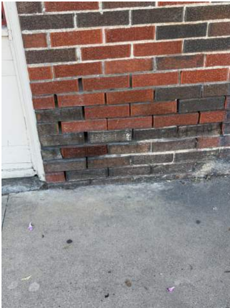
Figure 15. Gaps in the brick at the base of the facade where the brick meets the concrete foundation.
