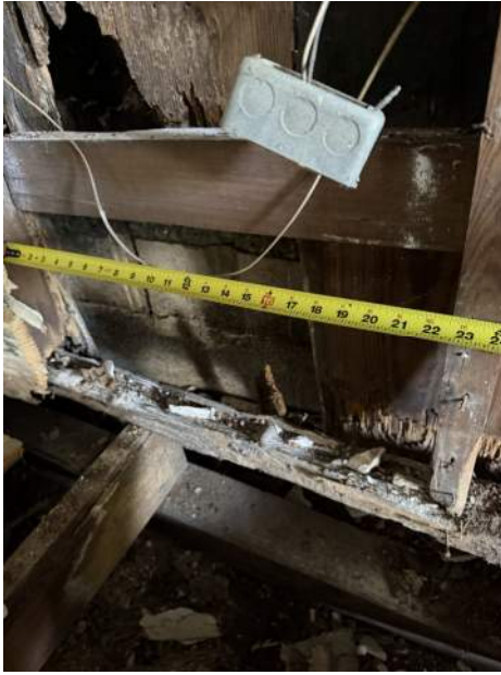
Figure 9. Bottom of the existing 2x4 bearing wall with floor joists bearing, adjacent to the neighboring building wall. The sill and stud bases are deteriorated.
