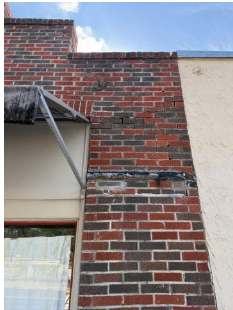
Figure 14. Stair-stepped separation at the brick mortar joints at the facade return – minor; possible indication of soil movement. No large cracks were observed in the facade.
