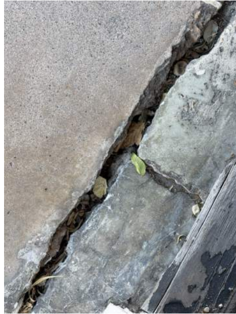
Figure 16. Crack in the front wall foundation at the doorway, and separation between the sidewalk and the front foundation.
