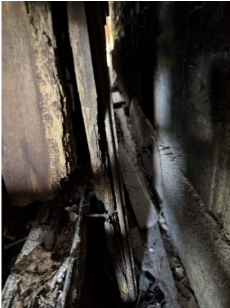
Figure 11. South wall base deterioration at the adjacent building – moisture infiltration through the gaps in the siding.
