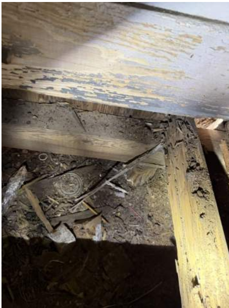
Figure 7. Deteriorated 2x6 floor joists at 24 inches on center bearing on the timber beam and pile foundation.
