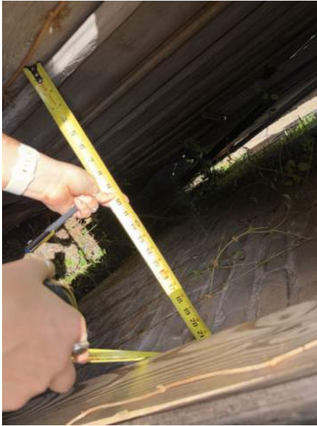
Figure 3. Gap between the existing 2x4 north bearing wall and the adjacent building to the north – approximately 21 inches. Water drains through this gap and toward the building.
