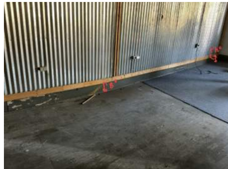
Figure 8. Approximate variation in floor height at the sinking floor – the markup shows the distance from the floor to the horizontal wall member, approximately 8 inches near the middle of the building and approximately 5 inches toward the end of the wall. The difference is the approximate floor depression of 2 to 4 inches.
