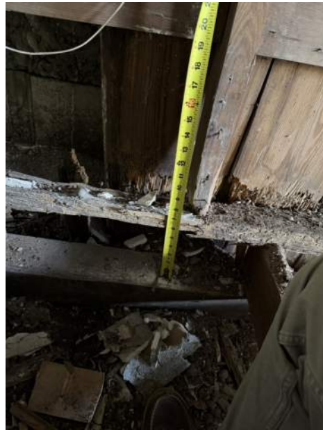
Figure 10. South wall – deteriorated wood wall construction. Splits and section loss at the base of the 2x4 studs.
