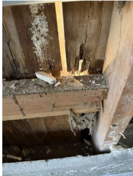
Figure 12. North wall – interior deterioration and water damage at the sill and stud bases.
