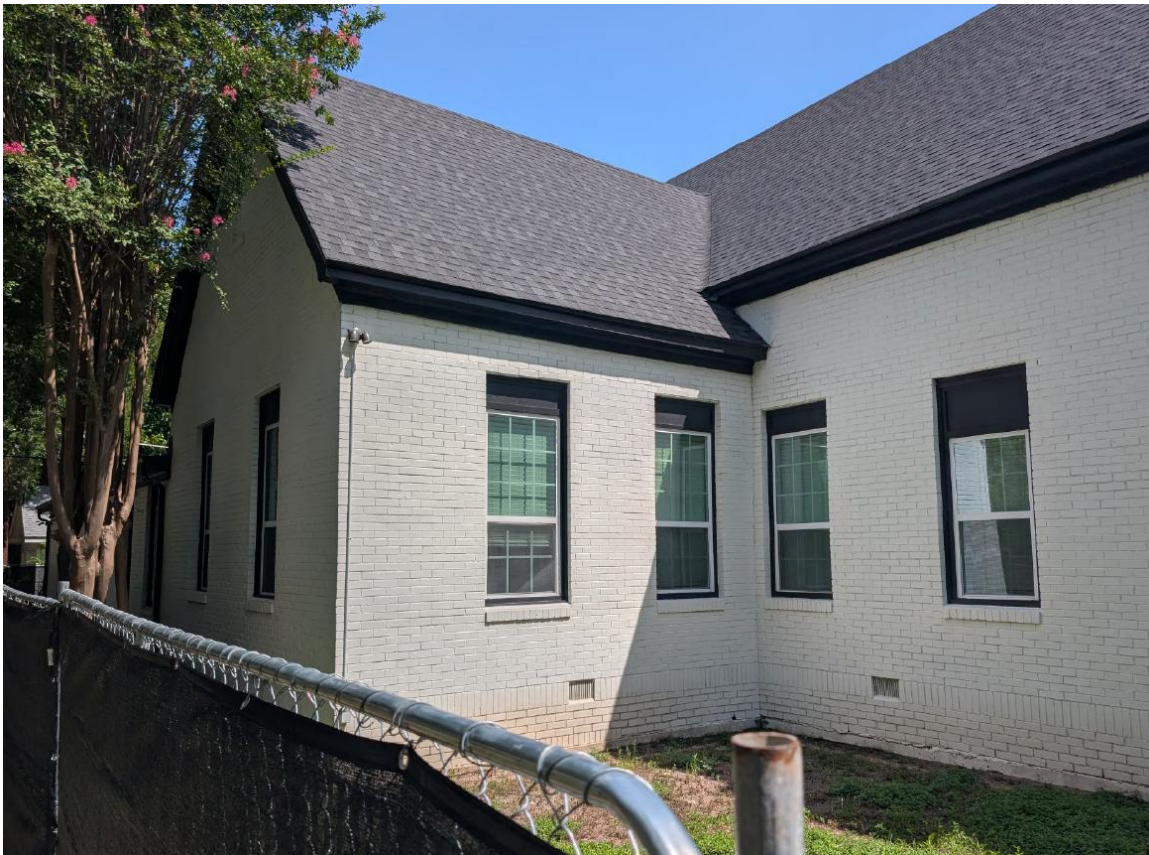
Site visit photos, 2026. Windows have been replaced with fixtures that do not fit their openings.
