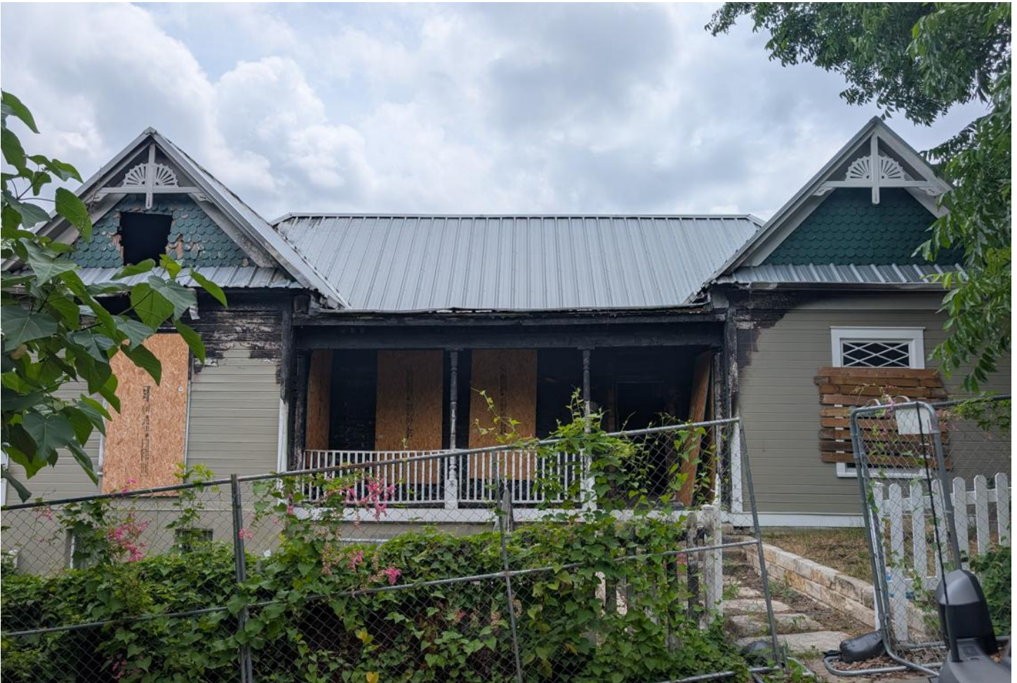
Site visit, showing fire damage (see backup for additional photos), May 2026
